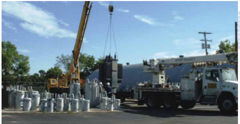
Wyrulec crews help guide the 14,700-lb. transformer onto a flatbed to move it to the Lingle substation. A boom crane from Scott & Son in Torrington was both available and big enough to do the moving job.
